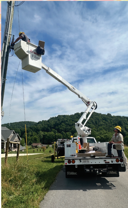
Building connections: A bucket crew hanging a new Network Access Point (NAP) to enable splicing for customer drops and expand service capabilities.
