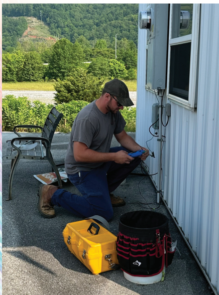
Final connection: A splicer meticulously working to splice the drop fiber to the NID on the side of the house, bringing reliable fiber service directly to the customer.
